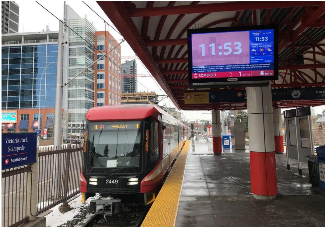
Figure 1: NANOV 55" Single-Sided Passenger Information Display Signs (PIDS) attached to canopy at Victoria Stampede CTrain Station in Calgary, Alberta
