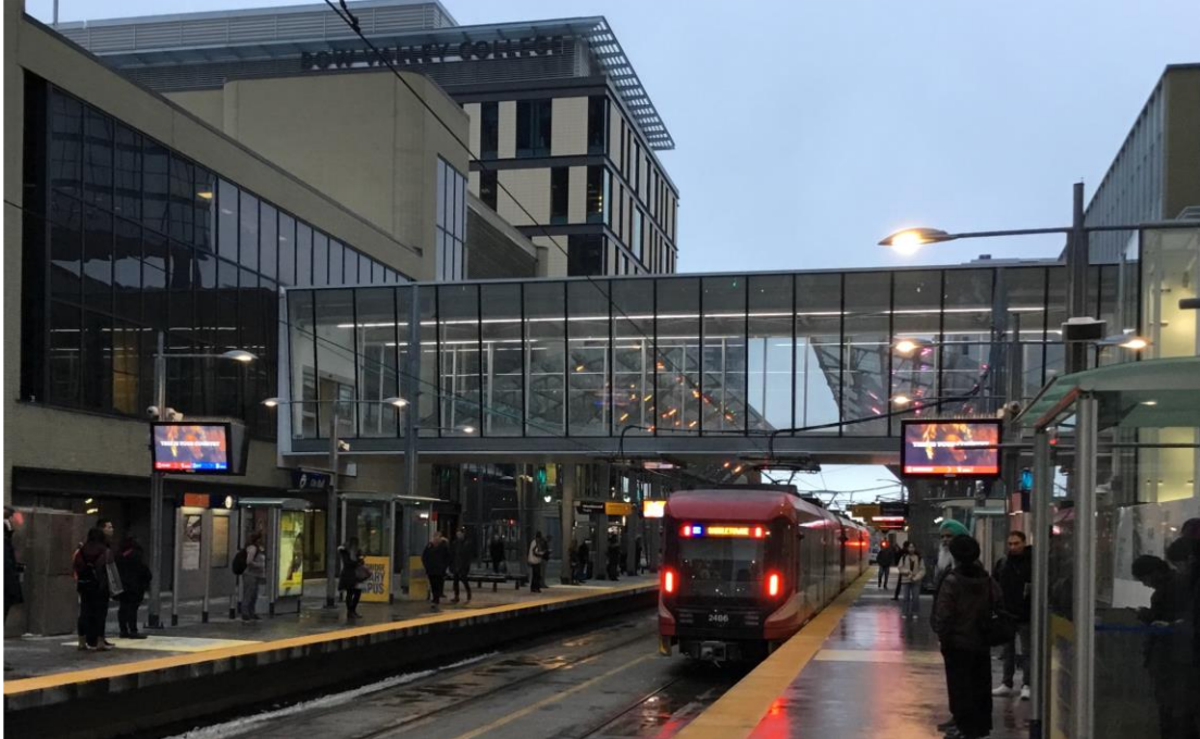
Figure 5: NANOV 55" Single-Sided Passenger Information Display Signs (PIDS) attached to lamp posts at CTrain Station in Downtown Calgary
