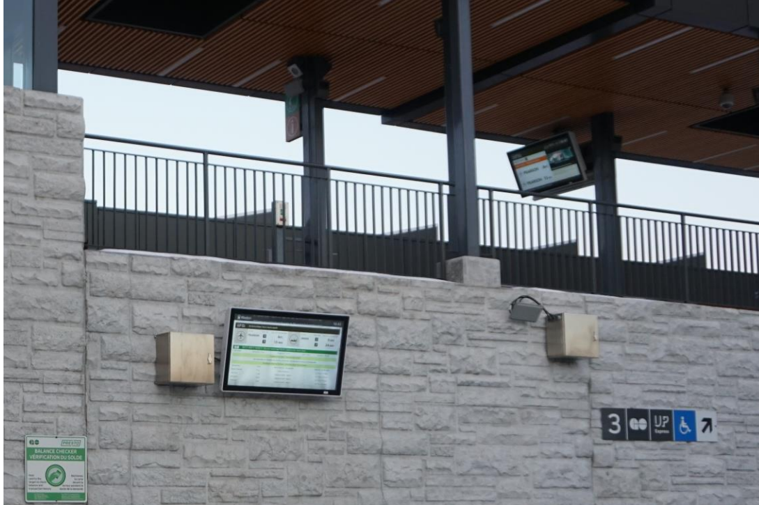
Figure 6: NANOV 46" Outdoor Real-Time Single-Sided Transit Signs featuring ceiling and wall mounts at GO Transit & UP Express Weston Station in Toronto, Ontario.
