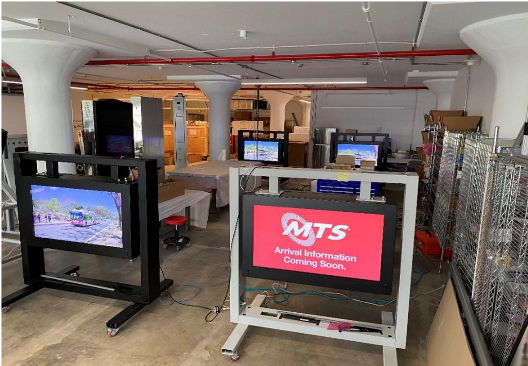
Figure 5: Integration and Commissioning of SDMTS Real Time VMS at NANO V R&D Facility in Brooklyn Navy Yard in Brooklyn, NY
