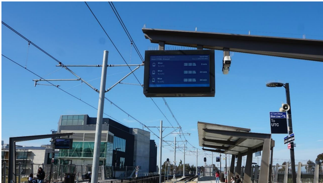
Figure 2: NANOV 46" Double-Sided Real Time Variable Message Sign (VMS) in San Diego Blue Line Station
